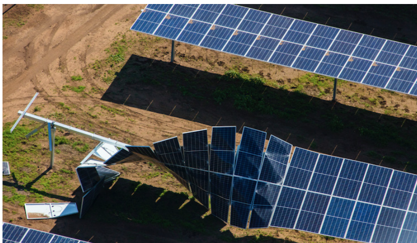
Figure 1 — Damaged modules at the Oakey 2 site in 2018. 5
