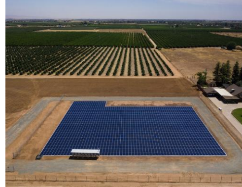
656 kWdc: Tulare County, CA COD: July 12, 2022
