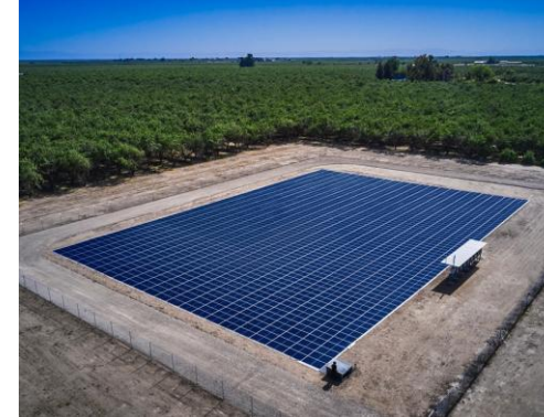
616 kWdc: Madera County, CA COD: May 25, 2022
