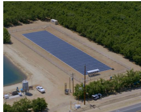
336 kWdc: Kern County, CA COD: August 6, 2021
